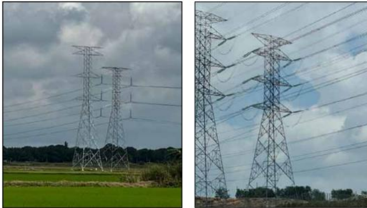
Lattice pylon towers
